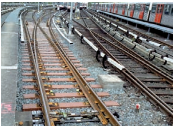
The modular turnout with synthetic sleepers was installed at HHA's Farmsen depot in less than one day.
